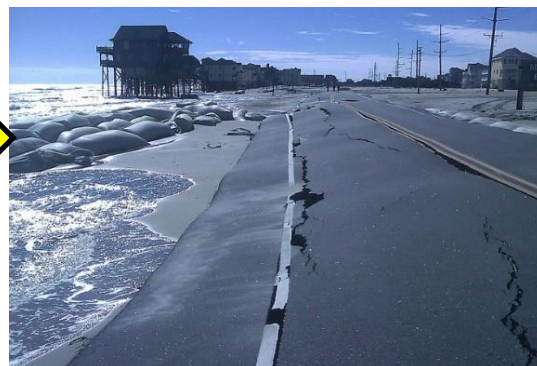
Potential application to prevent similar scenarios: Mirlo beach after ineffective sandbag protection [c]
