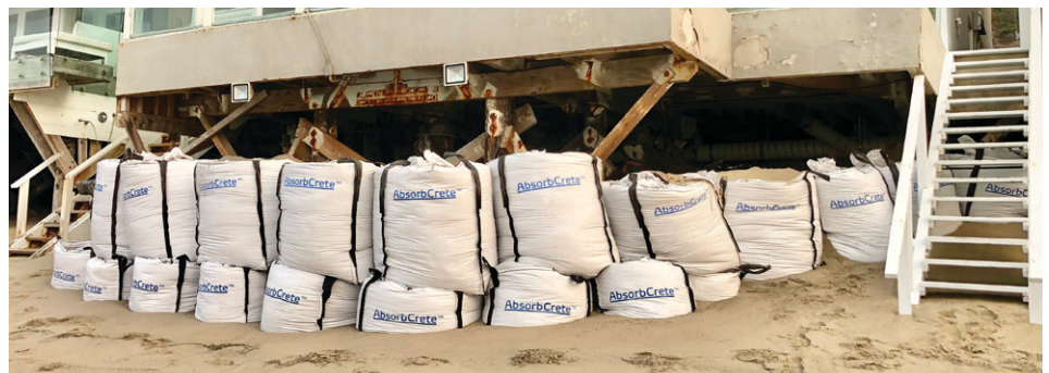
Figure 1. Absorbcrete® FIB bags used for ocean tidal site protection – foundation repair, Malibu, California.
